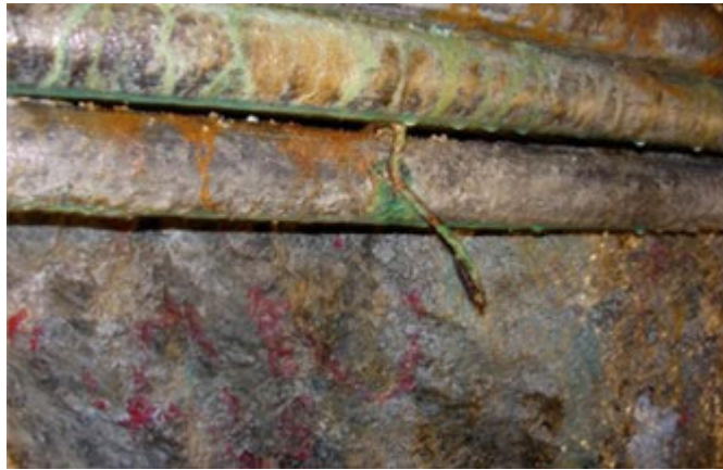
Figure 2 – Biofilm (that can increase corrosion problems) over a pipeline.
